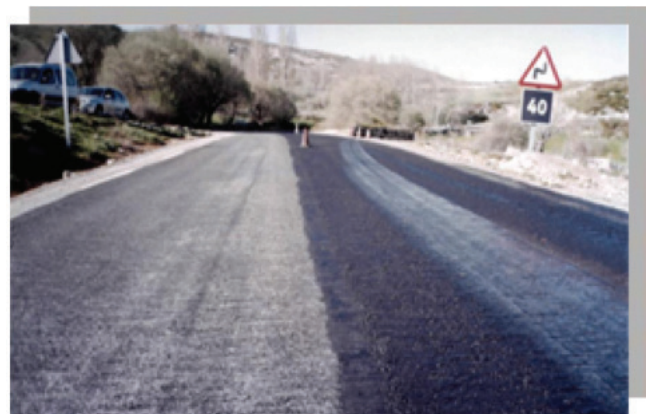
Construction of anti-icing pavement with AIA in the mountainous region of Avila, Spain
